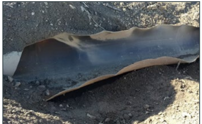
Figure 9: Overall view of the fractured line
