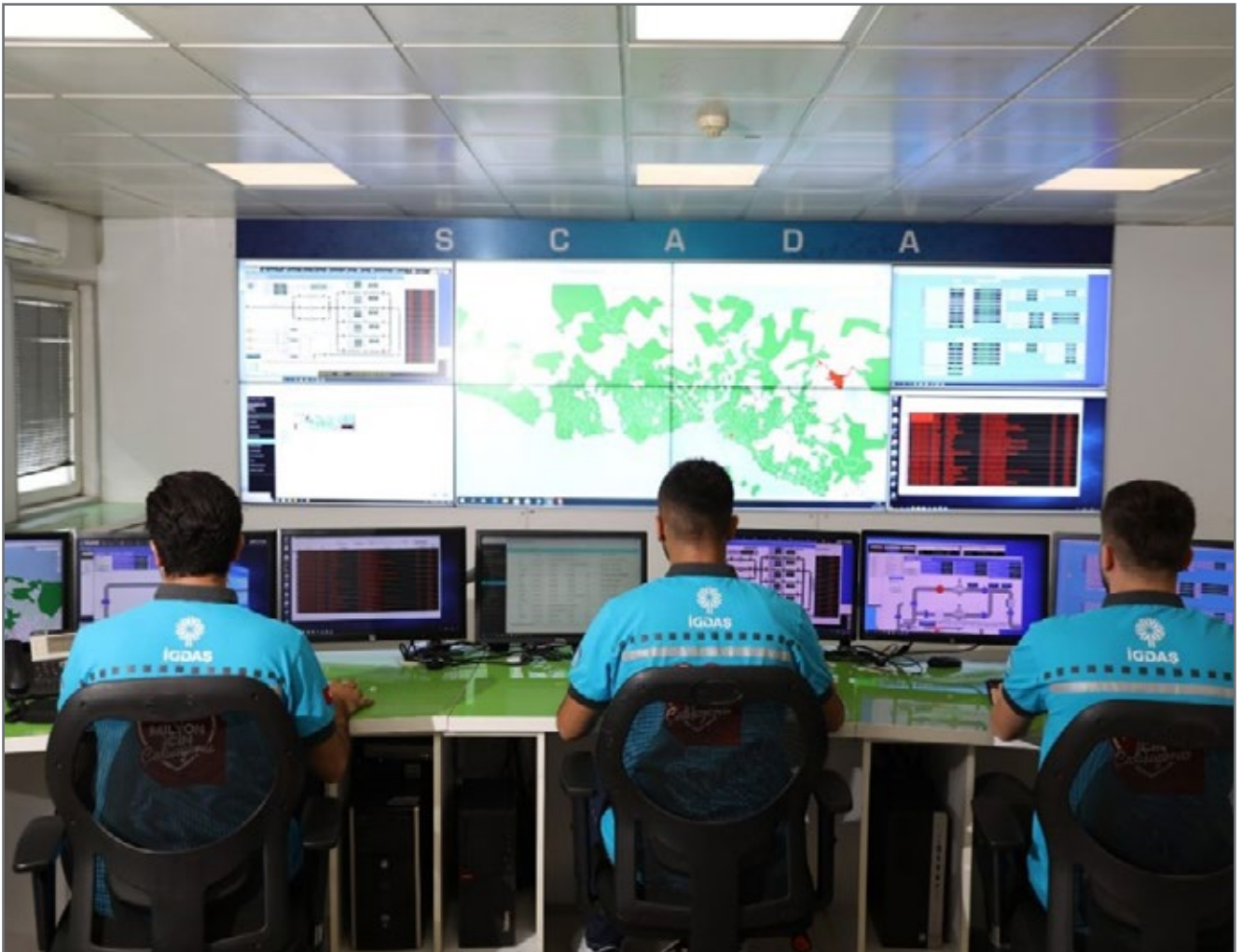
Figure 2: SCADA Control Room
