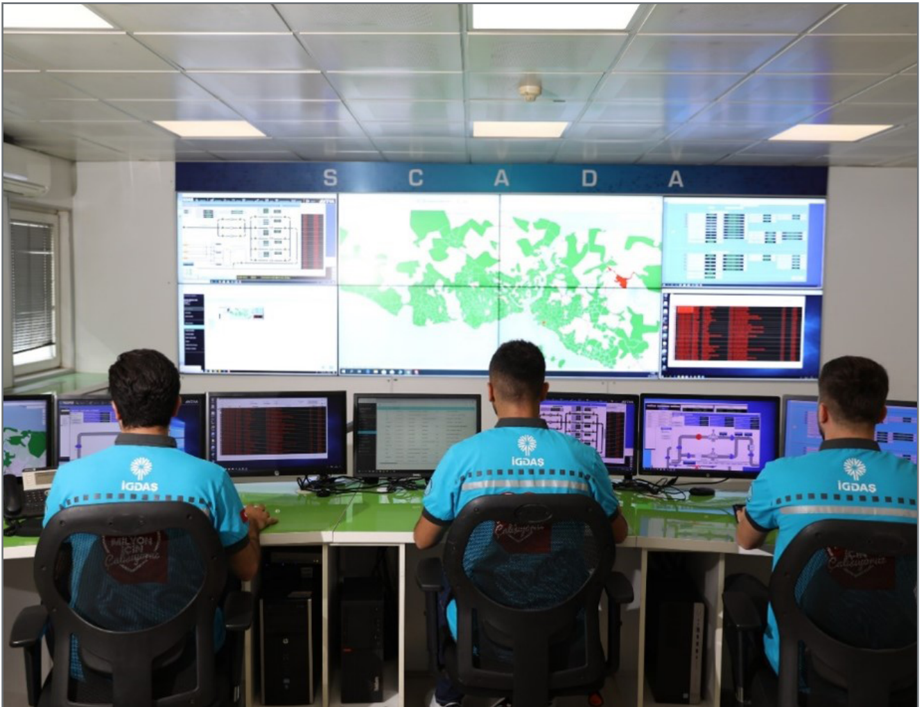
Figure 2: SCADA Control Room
